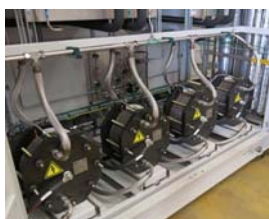
Fig. 6. 300 kW PEM water electrolyser (collaboration ArévaH 2 Gen).
