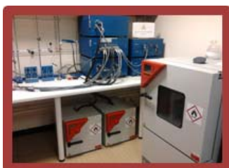
Fig.19. Batteries cycling room facilities.
