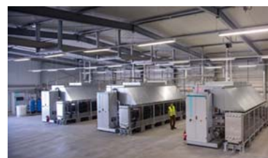
Fig. 7. 7-MW PEM water electrolysis platform at EnergiePark, Mainz, Germany (collaboration Siemens).
